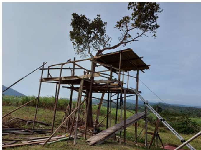
The beginning of the construction of the TREE CAMP - July 2020. Completed skeletal structure for the TREE Gallery.
